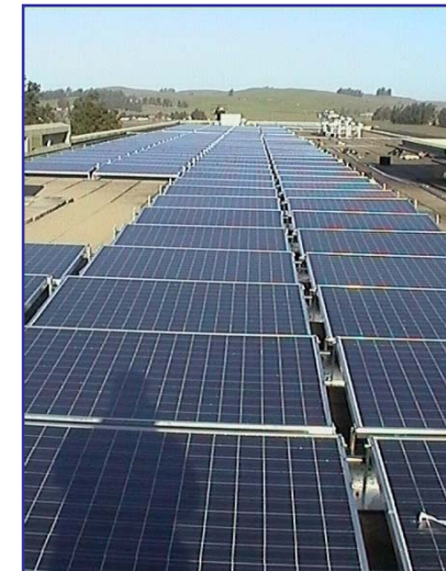
Photovoltaic Array, TRACEN, Petaluma, CA
